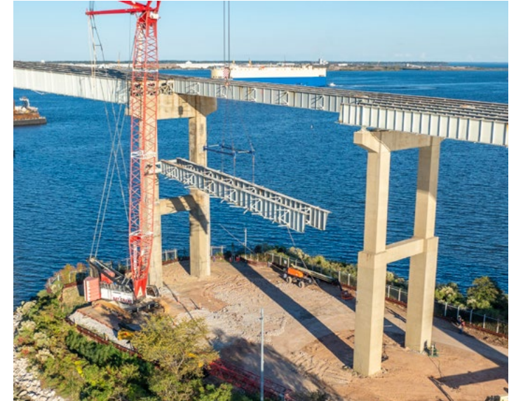
▲ The removal of the first steel girder on the south side of the bridge.
