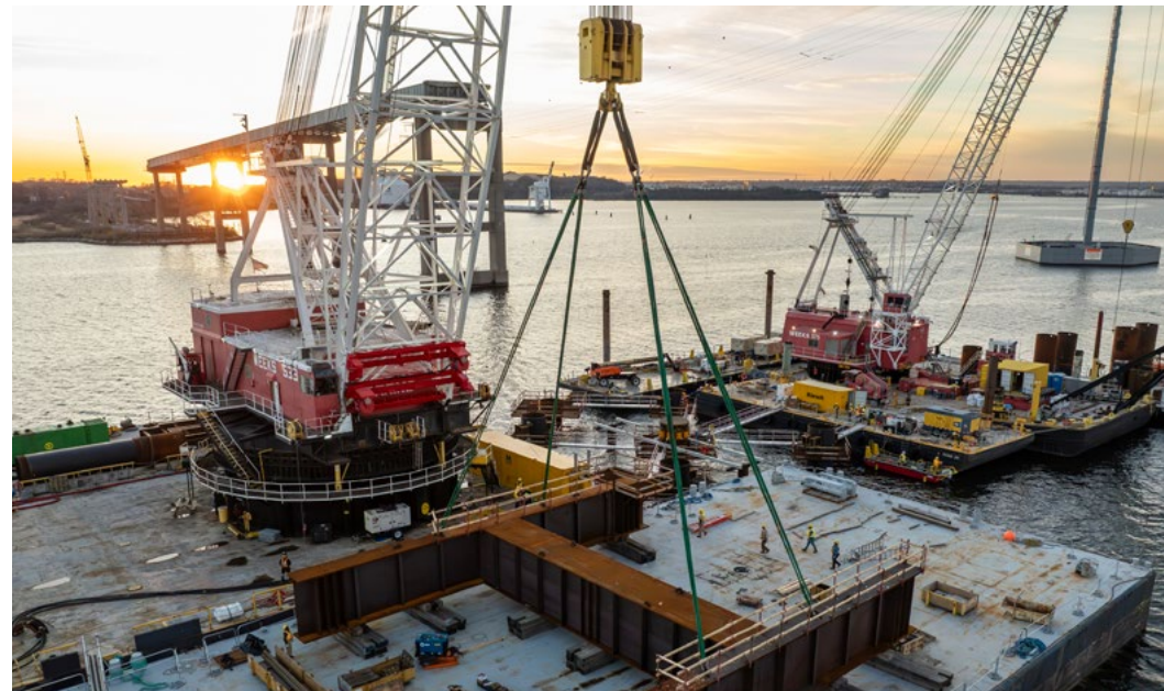
▲ Weeks 533 crane preparing to lift the load frame and place it on the test piles.
